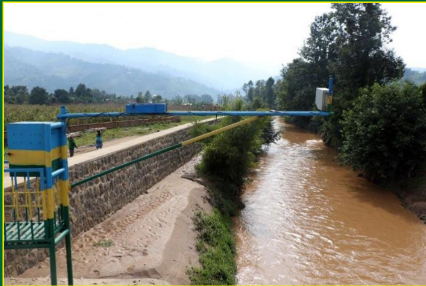
Early warning system installed at Sebeya River
